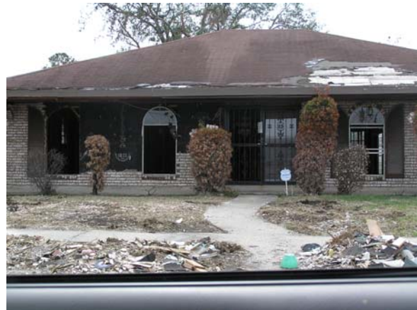
Figure 12. Wind damage to neighborhood buildings
