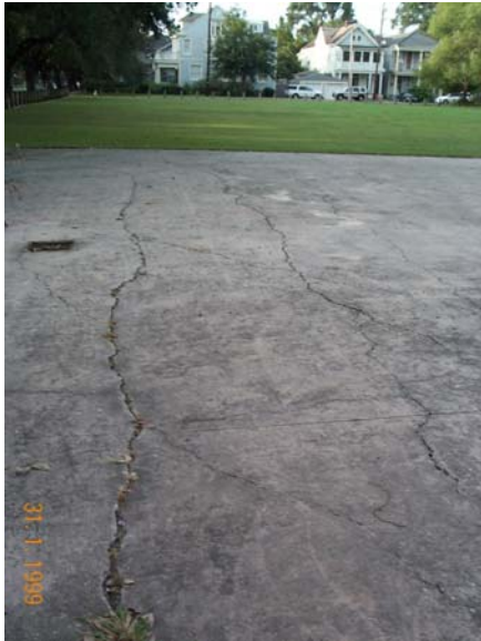
Figure 62. Deduct points on condition of court surface for cracks.
