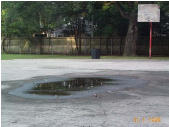
Figure 63. Deduct points for surface unevenness, allowing standing water, and cracks.
