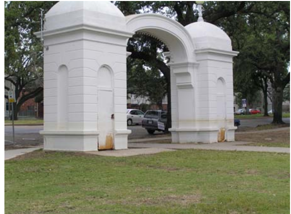
Figure 4. Evidence of flooding in park (note flood lines)
