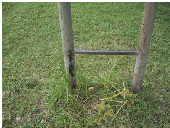
Figure 91. Deduct points for corrosion.
