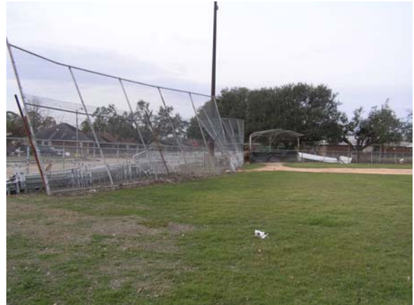
Figure 8. Damage to play/sports equipment
