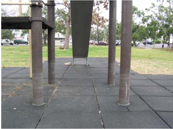
Figure 3. Evidence of flooding in park (note flood lines)
